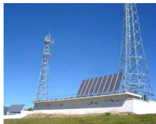
communication base station
